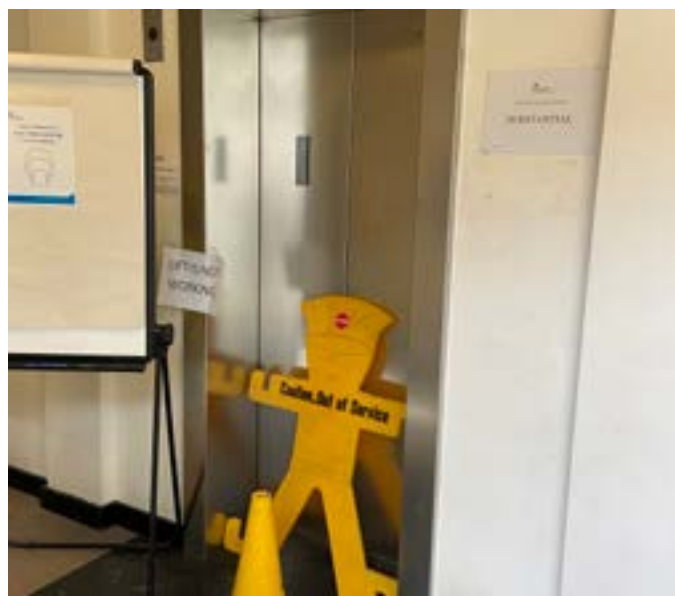
Lift in need of repair at a court building
